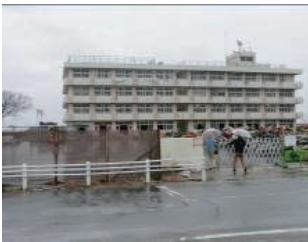
Damage to Arahama Elementary School
