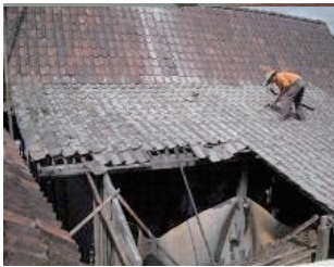
Roof and building damage due to Merapi Eruption in 2010
