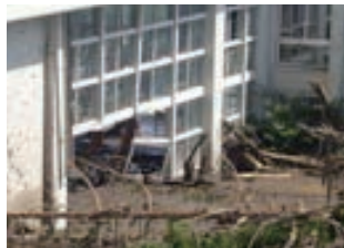
Debris flow at the Uenohara Elementary School
