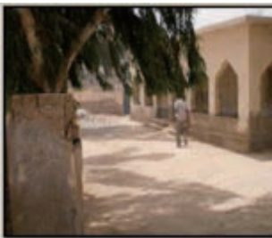
Partially Damaged School
