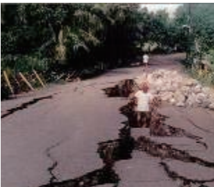
Some roads in Dagupan became impassable
