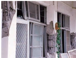
Damage to a building of Tong-Lin Elementary School
